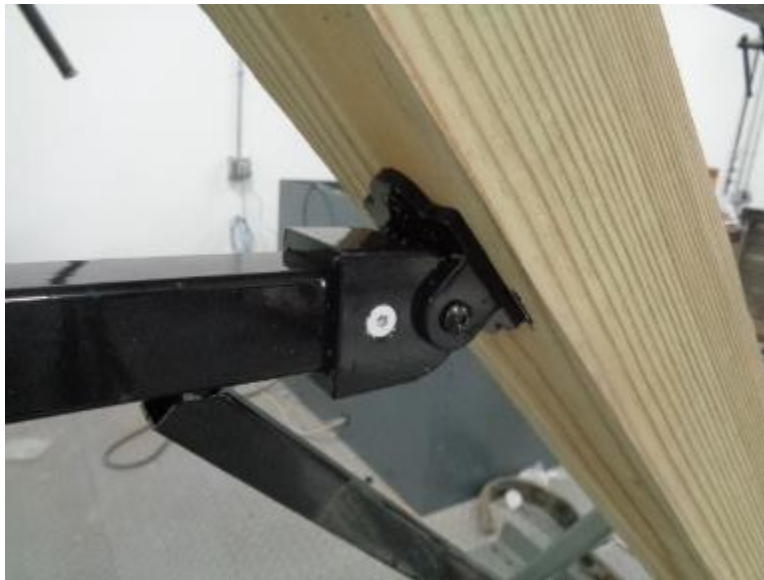
Photo No. 7 Stair Bracket Attached to Wood Post
